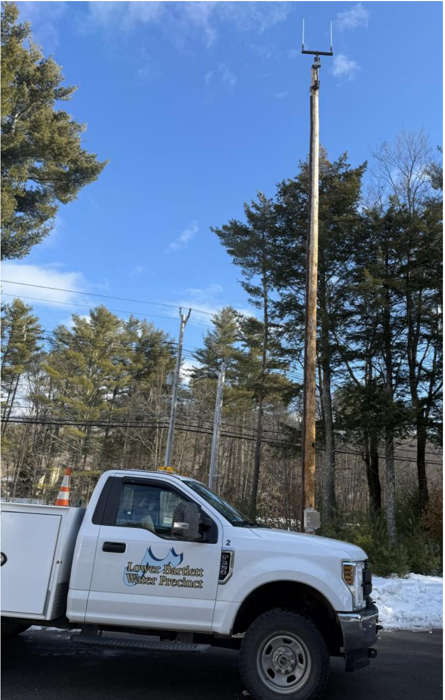
Lower Bartlett Water Precinct truck in front of one of their AMI collectors.
