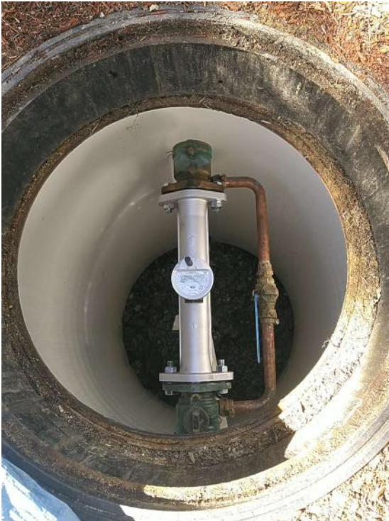
Meter location in a pit.
